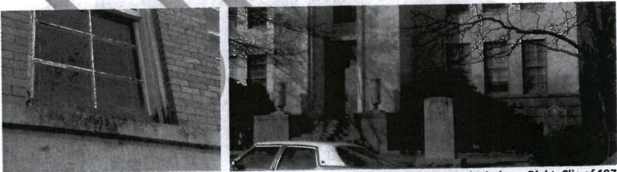
Left: Example of failing paint and biological growth at cast stone sill below deteriorated window. Right: Clip of 1975 photograph showing cast stone base painted green.
