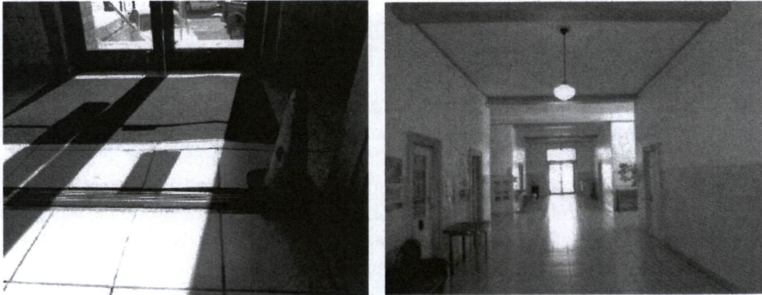
Photos of corridor floor tile that has been removed. Courtesy of Randall Scott Architects.
