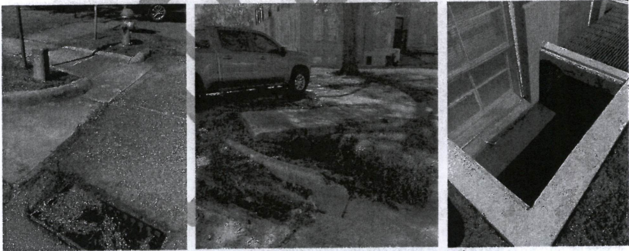
Left: Stormwater grate at southeast corner. Center: Culvert at northeast corner. Right: Example of standing water in areaway.
