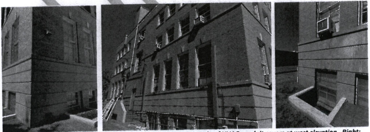
Left: Mini split view with visible condensate drip. Center: Example of HVAC conduit covers at west elevation. Right: Example of window unit with visible condensate drip.
