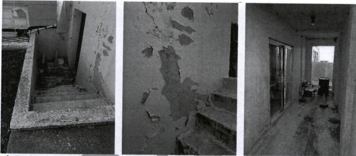
Left: Basement stairs at northeast side. Center: Severe paint peeling at porch wall adjacent to basement stair. Right: View of north basement vestibule.
