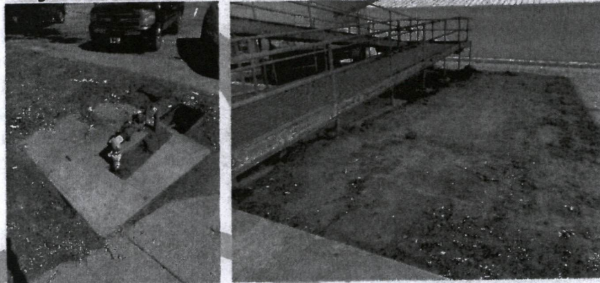
Left: Water main, note new PVC. Center: Saturated soil at northwest side of Square.
