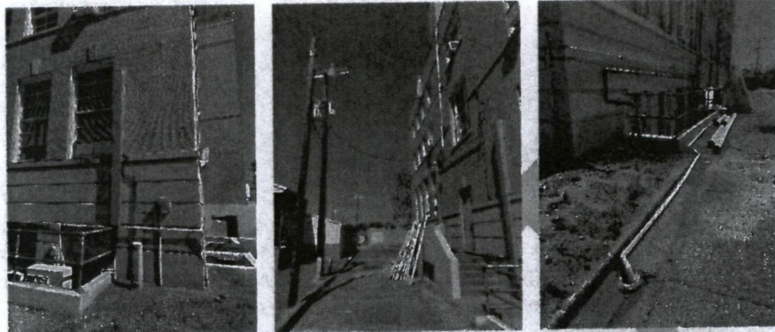
Left: Example of mini split cassette at areaway and intrusive exterior conduit covering. Center: Overhead powerlines entering building at west elevation. Right: Exposed water supply at west elevation entering boiler room.
